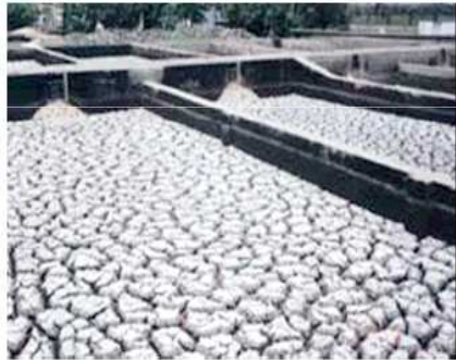
Figure 2: Large lumps in overfilled drying beds (source: ipp consult )
