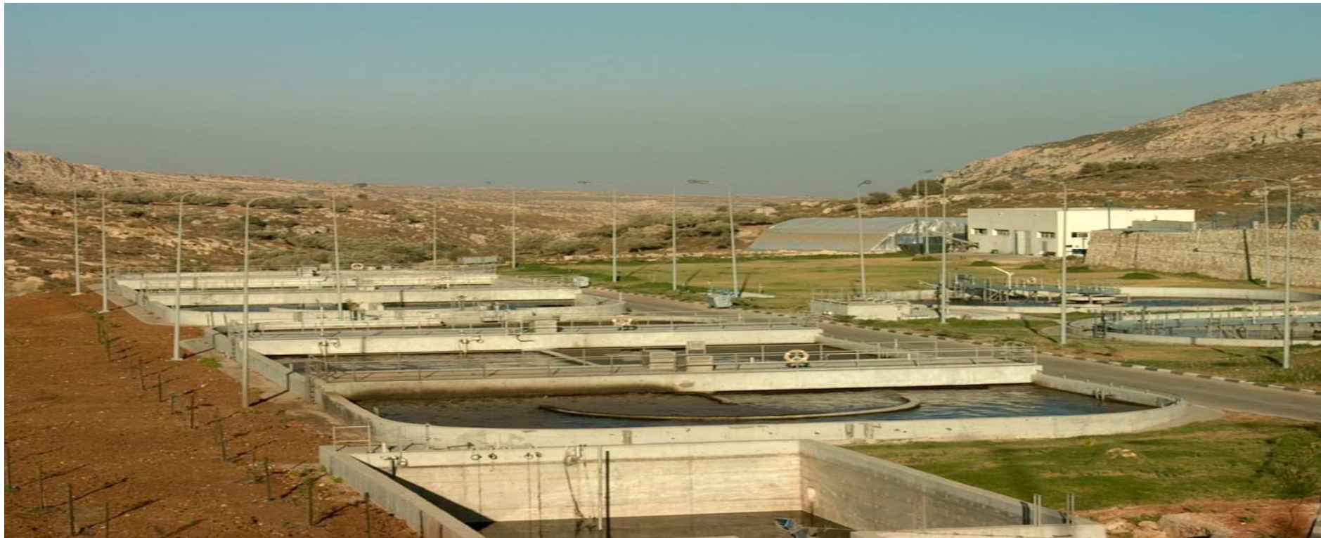
Al-Bireh wastewater treatment plant
